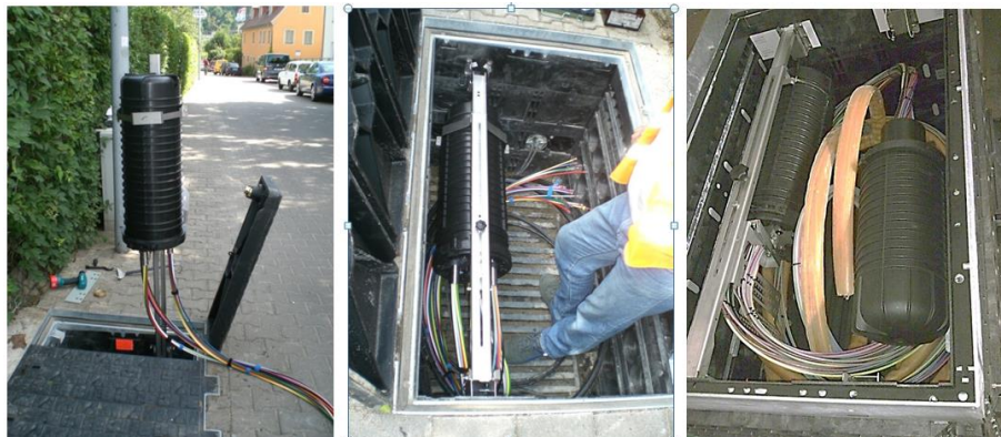
Figure 13: Underground fibre distribution with closures
